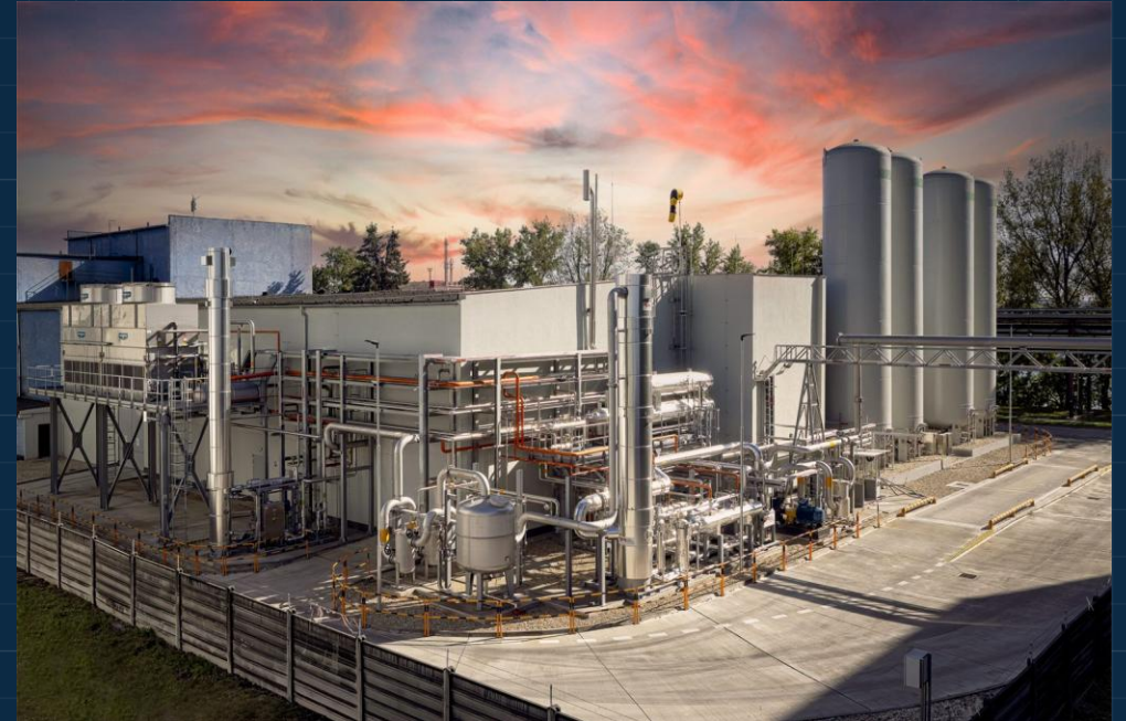
FIG. 01 — CO 2 recovery plant, SIAD Slovakia, Leopoldov · process plant designed and supplied abroad; IPE: documentation audit, approval inputs and permitting for trial and permanent operation, 2022–2024. Photo: SIAD Slovakia.
